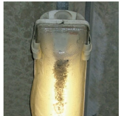
Compromised IP rating
